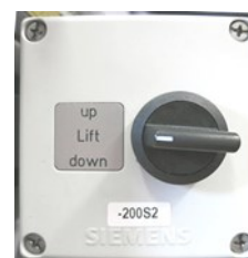
Switch of the lift system
