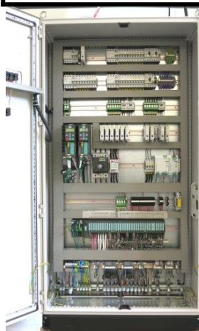
Switching cabinet (inside)
